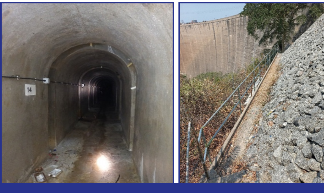
Figure 21. Refurbished lighting circuits and fittings in Adit 1392 and new handrails on the north bank access to gallery F.
