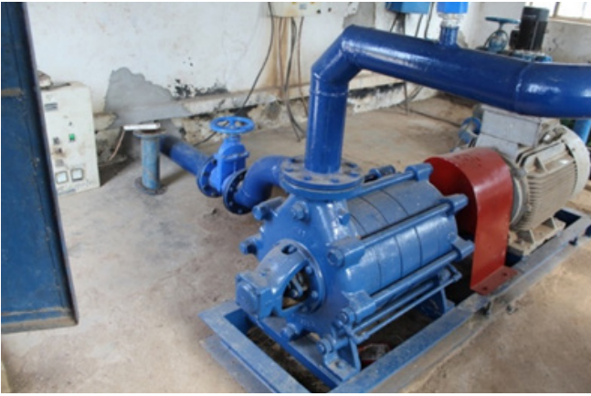
Figure 26. A newly installed gate valve and suction line at Pambazana Booster Station in Chirundu
