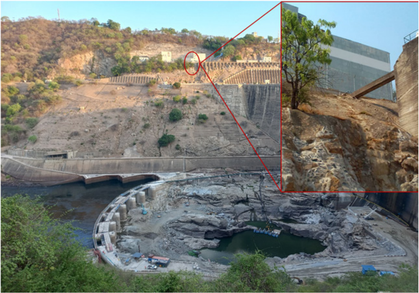
Figure 22. The south bank slope and plunge pool. The insert shows the typical surface protection repairs of the surface by stone pitching.
